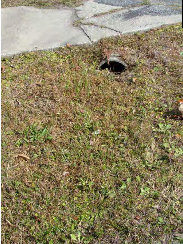
Photo 5— Stormwater drainage problems
