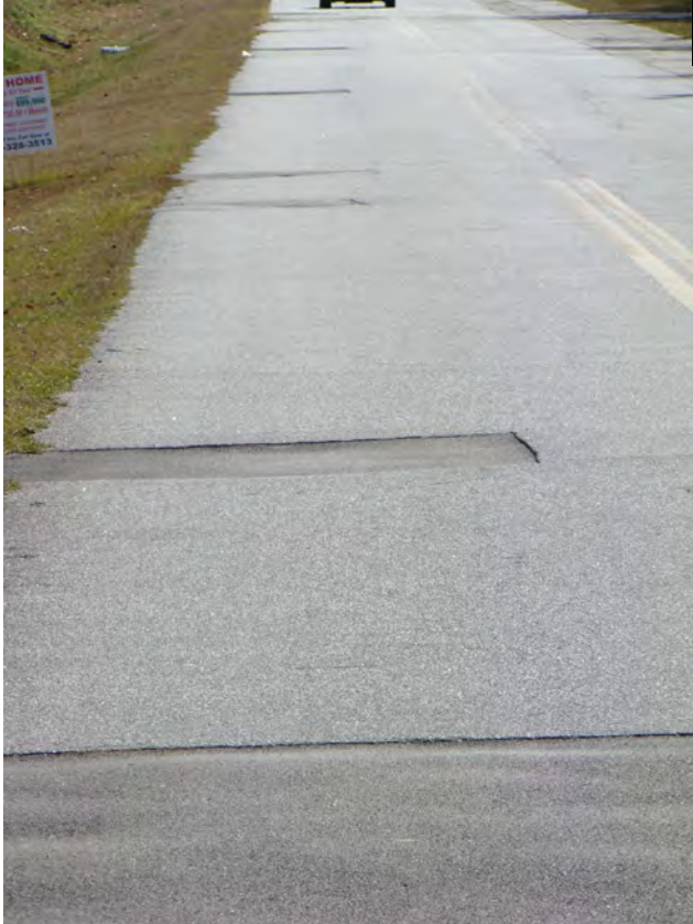
Photo 9 — Roads in need of repair
